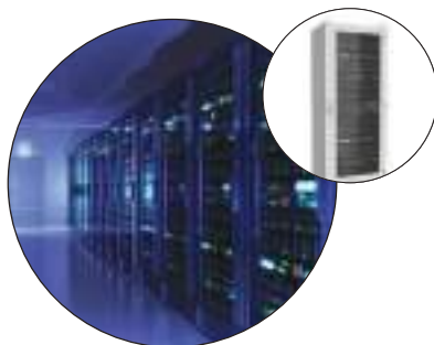
Telecom and Computer
